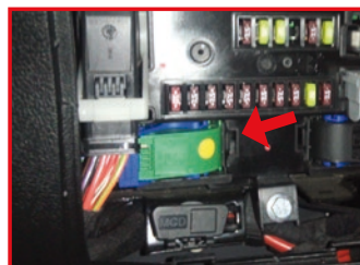
Green plug in fuse box on Fiat Ducato platform (Type 250/290)
